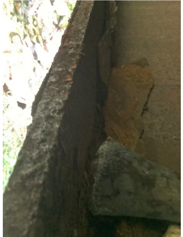
Rust scale ds right abutment. Inside ds girder. Typical.
